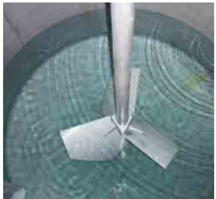
Maturation mixers - wastewater treatment
